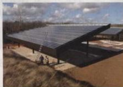
The three new solar arrays at the North Carolina Zoo are complete and generating power. One array and shelter is obscured in this view.
